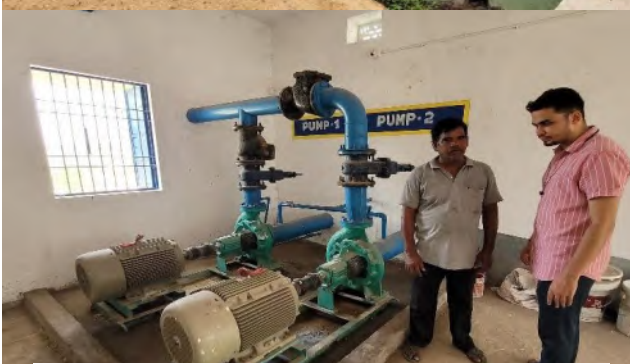
Pump House at Santhapada
